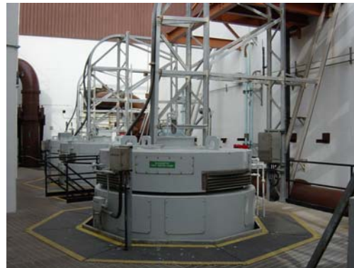
Using SensiNet® to Monitor Temperature in Water Circulation Pump Motor
